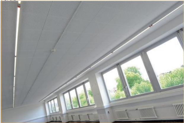
View of an office wing: Especially the low installation costs, the absence of flickering and the good light quality are convincing arguments for the long-term lighting concept. Non-glaring and pleasant, healthy light enable fatigue-free working.
